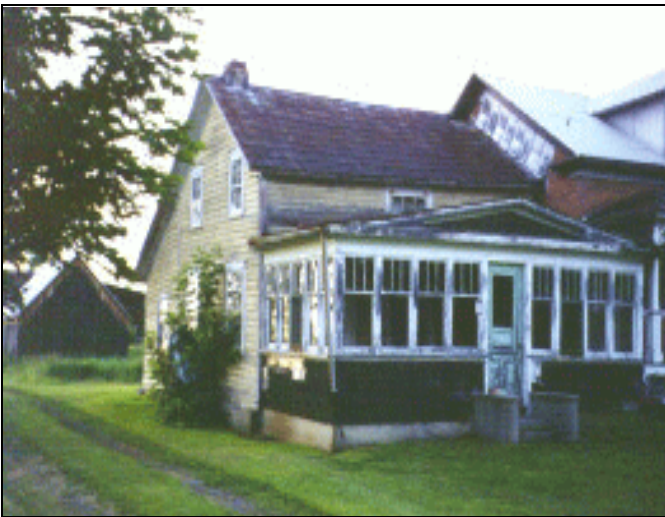
Figure 1: Frost walls on older homes were typically not deep enough to prevent frost heave and sagging foundations
