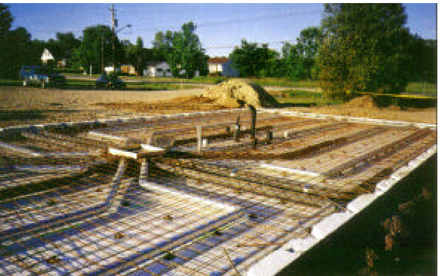
The insulating form (top) is set in a mortar bed. Centre, a layer of 6" wire mesh is placed over the insulation. Then the heat distribution box and ducts are laid out (bottom).
