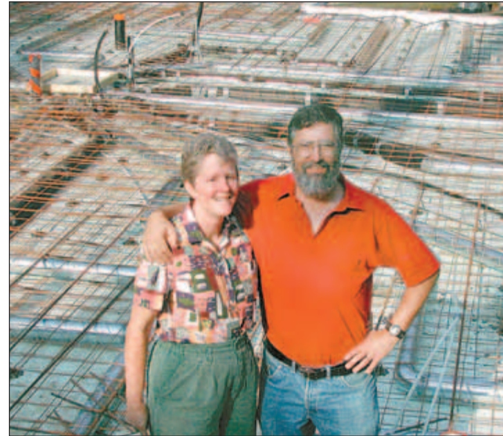
Kathleen Pickard and Arthur Ham's Ottawa River home will rest on an innovative Legalett slab foundation made of Styrofoam.
